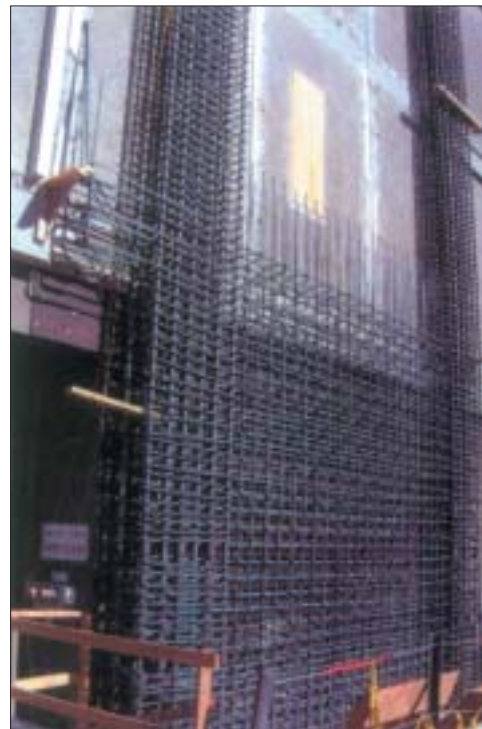
High volume Fly Ash has been used in the Barker Hall Project, University of California at Berkeley for the construction of shearwalls.
