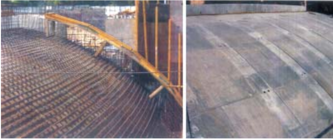
SCC poured at Rotary Dome at central secretariat station – Delhi Metro Project
