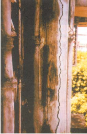
Crack formed due to bursting pressure on account of rusting of reinforcements
