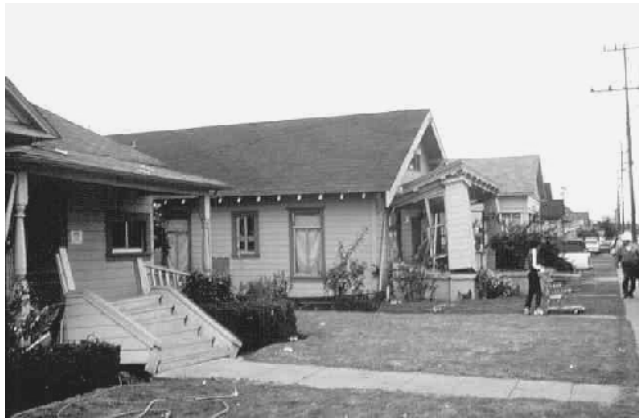
FIGURE 7.5 Houses damaged due to cripple wall failure, 1983 Coalinga Earthquake (courtesy of EQE International).
