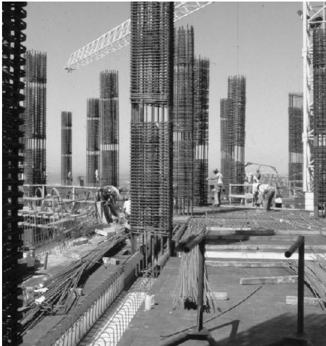
PHOTO 4.2 Installation of reinforcing bars in the Pacific Park Plaza building (courtesy of Mr. James Tai, T.Y. International, San Francisco).
