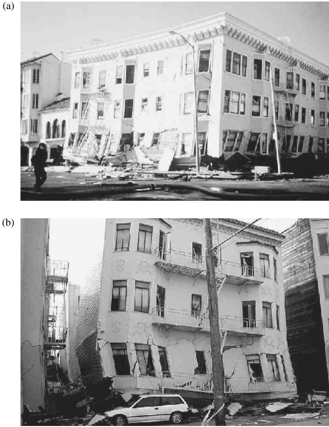
FIGURE 7.6 Collapsed apartment buildings in Marina district of San Francisco, 1989 Loma Prieta Earthquake (courtesy of EQE International).
