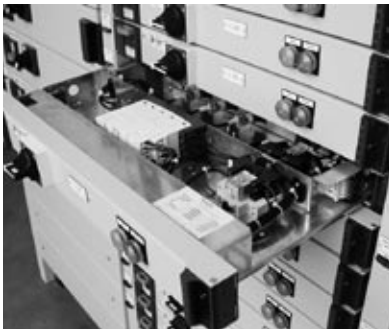
Fig. E32 : Distribution switchboard with withdrawable functional units in drawers
