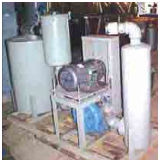
Blower driven by electric motor
