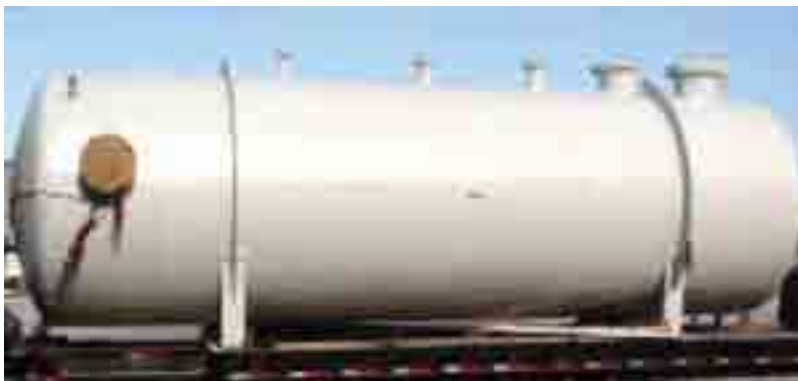
This vessel holds oil at high pressure.
