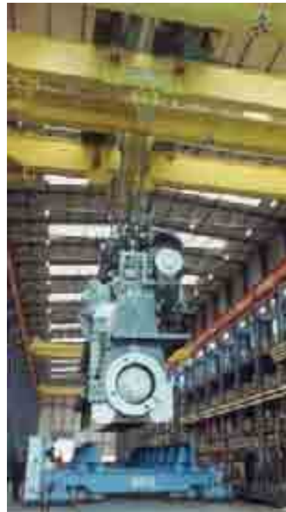
This heavy duty crane moves within shopfloor on fixed rails.
