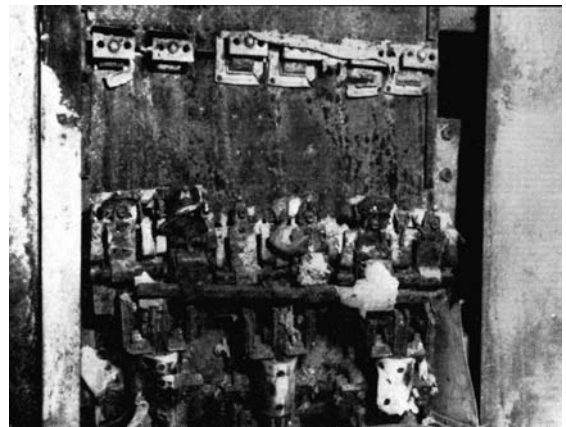
Figure 3 Fused feeder switch consumed by arcing fault in high-rise apartment main switchboard. No intermediate segregating barriers had been used in construction
