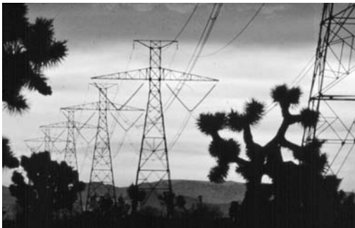
Figure 2 A \pm 500 -kV HVDC transmission line
