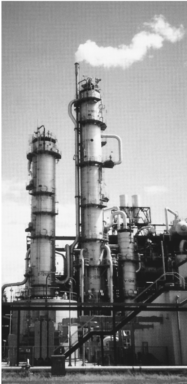
Fig. 6a. Distillation column (courtesy of Eickmeyer and Assoc.)
