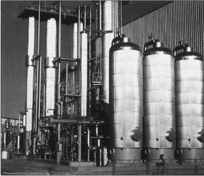
Fig. 5a. Pressure swing adsorption beds for the dehydration of alcohols ( courtesy of Howe-Baker Engineers )
