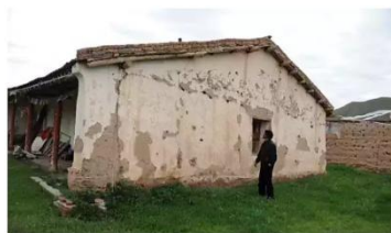
In the Tibetan plateau, a yak herder's home that has tilted and has been damaged due to thawing of the permafrost
