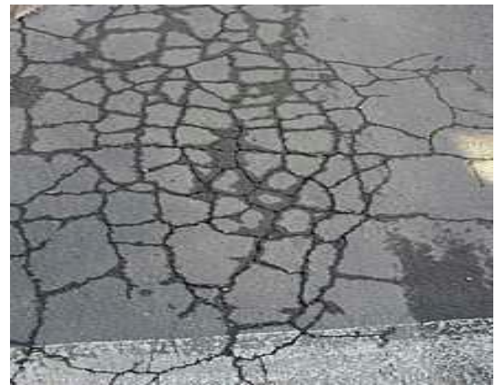
Fig. Map cracking
