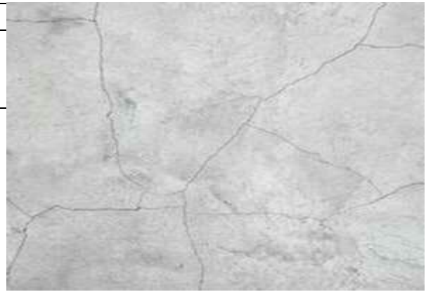
Fig. Plastic shrinkage cracking
